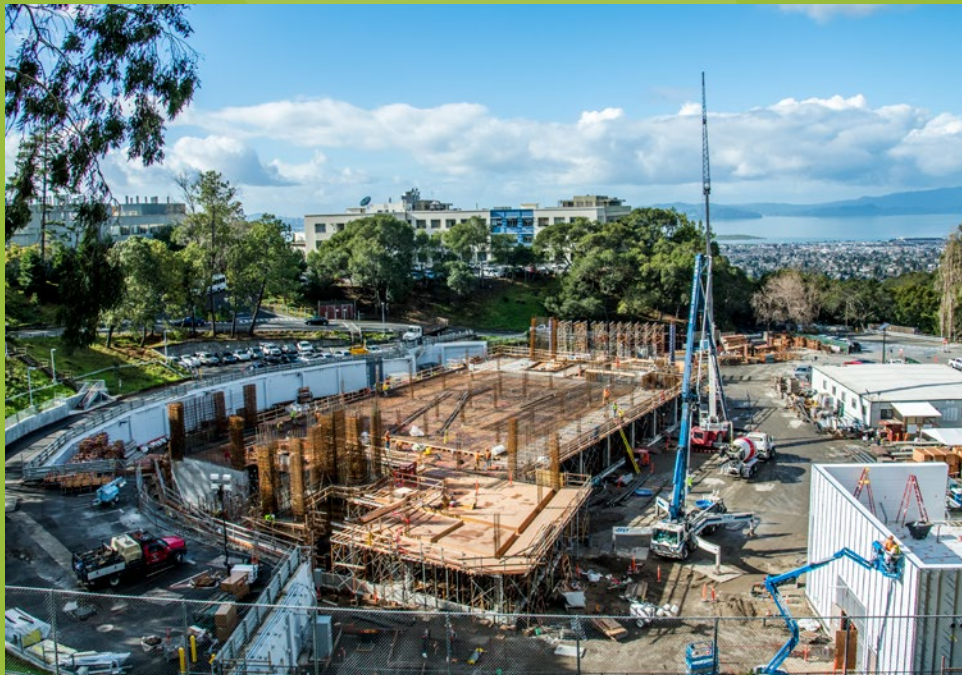
Ongoing construction of the Integrative Genomics Building (IGB) as of January 2018, future home of the JGI and KBase at Berkeley Lab.
