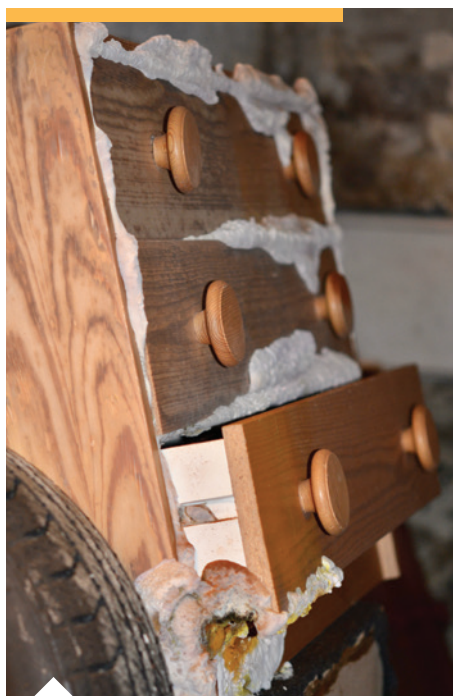
Dry rot attacking dresser. (Inger Skrede)
